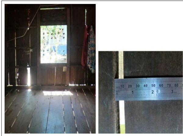
Figure 118 Floorboards with gaps.
